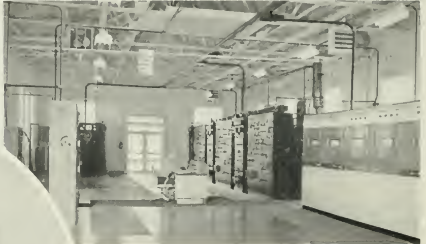
Interior of transmitter building showing high-frequency transmitters, in rear, and 500-kc transmitter (right). Frank Kremp, engineer-in-charge, at console.
